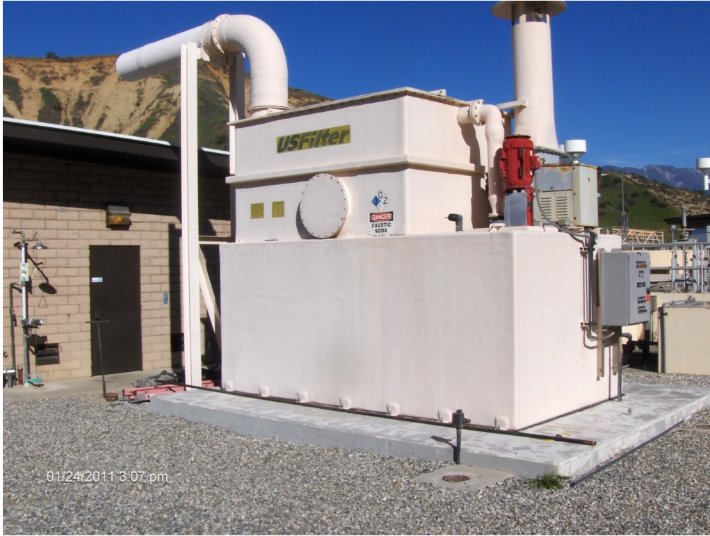
Emergency Chlorine Scrubber
