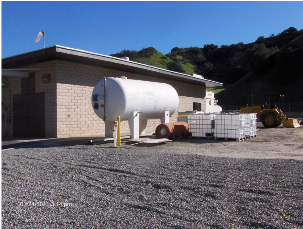
Aqueous Ammonia Storage Tank
