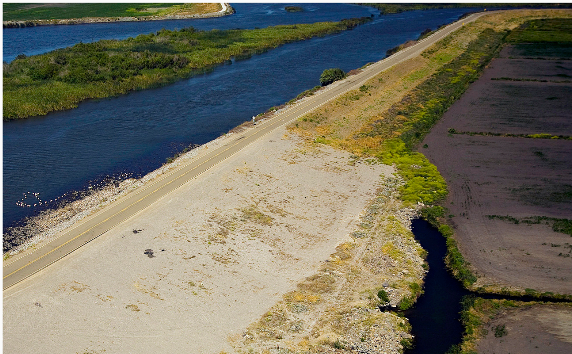
Subsidence (sinking) of islands in the Delta places even more pressure on already fragile Delta levees.
