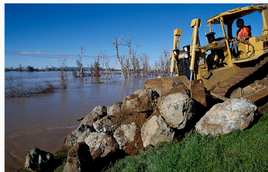
Many vulnerable Delta levees require installation of rock revetments, riprap, or other engineered structures along eroding banks to reduce erosion and protect levee foundations.
