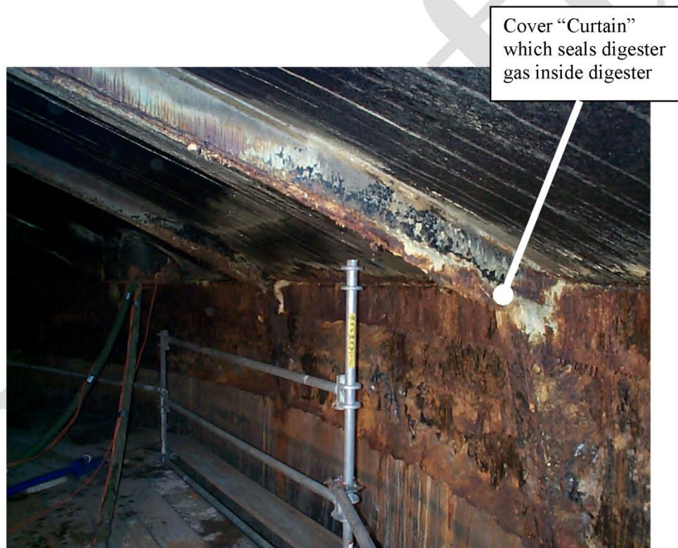
Figure 1 – Digester No 2 Cover Corrosion, Especially on “Curtain”
