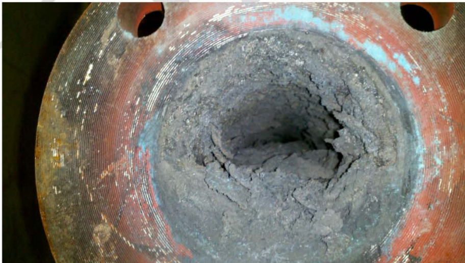
Figure 3 – Severe corrosion inside piping
