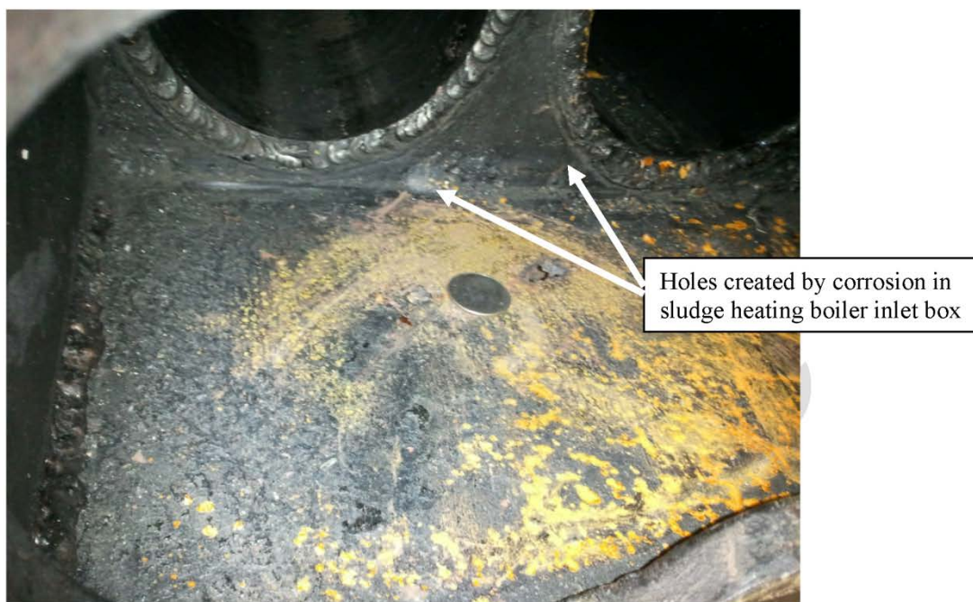
Figure 4 – Corrosion through inlet box base
