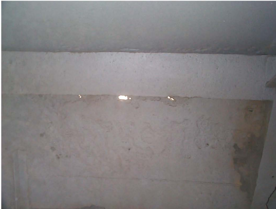
Figure 2 – Digester No 2 corrosion through cover, repaired in 2005
